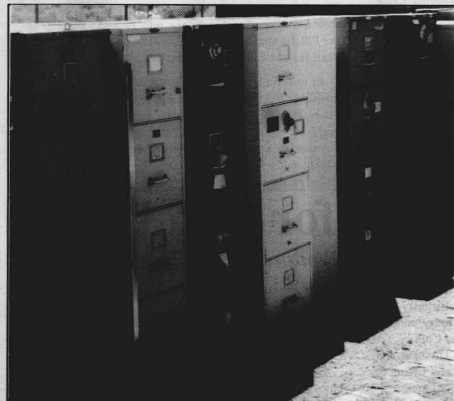
UNSAFES —Safes such as these manufactured by Remington Rand contain asbestos and must be disposed of properly... and quickly as the cost of disposal goes to $1,500 each after Nov. 30.
