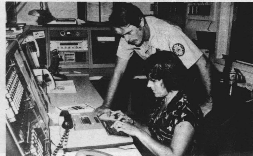
LIFESAVING DEVICE — Sheila Sauder, a consultant for the telephone company, shows Phil Sodergren, an NWC firefighter, how to use the new telecommunication device for the deaf that has been installed for the dispatchers in the Police and Fire Divisions so that deaf people can make emergency calls for help. The Fire Division's emergency number for the deaf is NWC ext. 3939; that of the Police Division is NWC ext. 3883.
